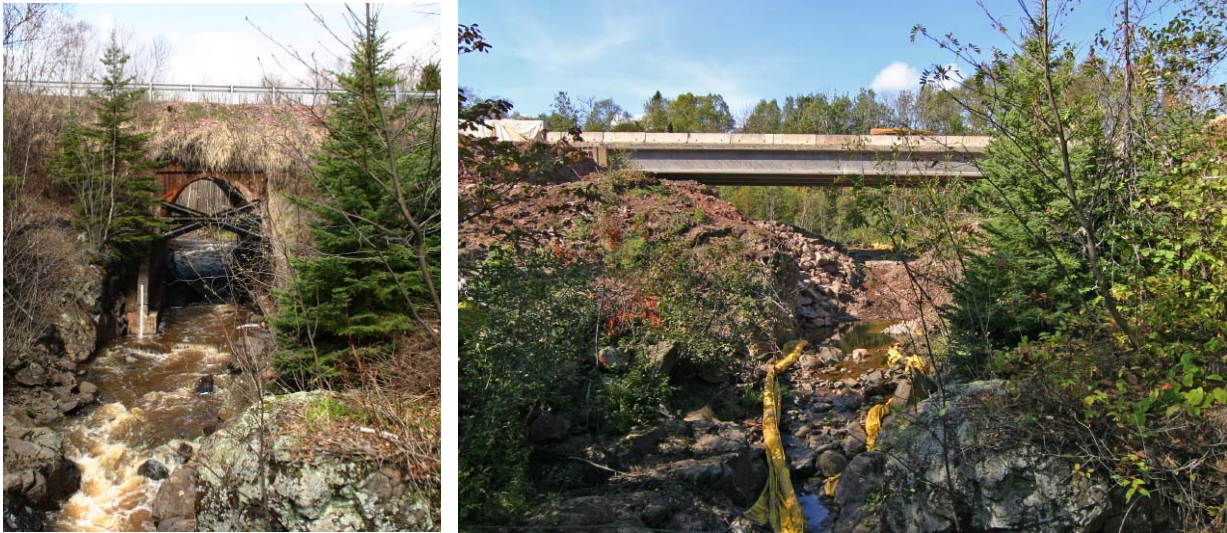
Figure 2. Example modification of a bridge to encourage wildlife use of an underpass. On the left is the original bridge, on the right is a widened bridge span with room for animals to cross underneath. Photo credit: Mn/DOT.
